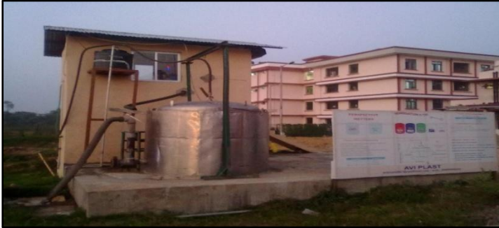
Biogas power plant at NIT Silchar
