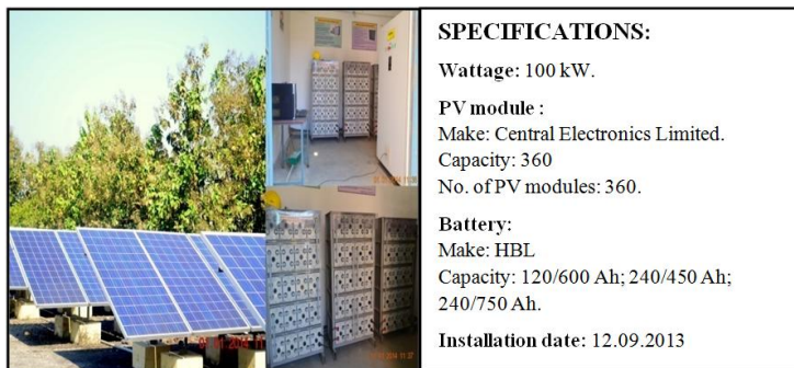
Solar power plant at NIT Silchar
