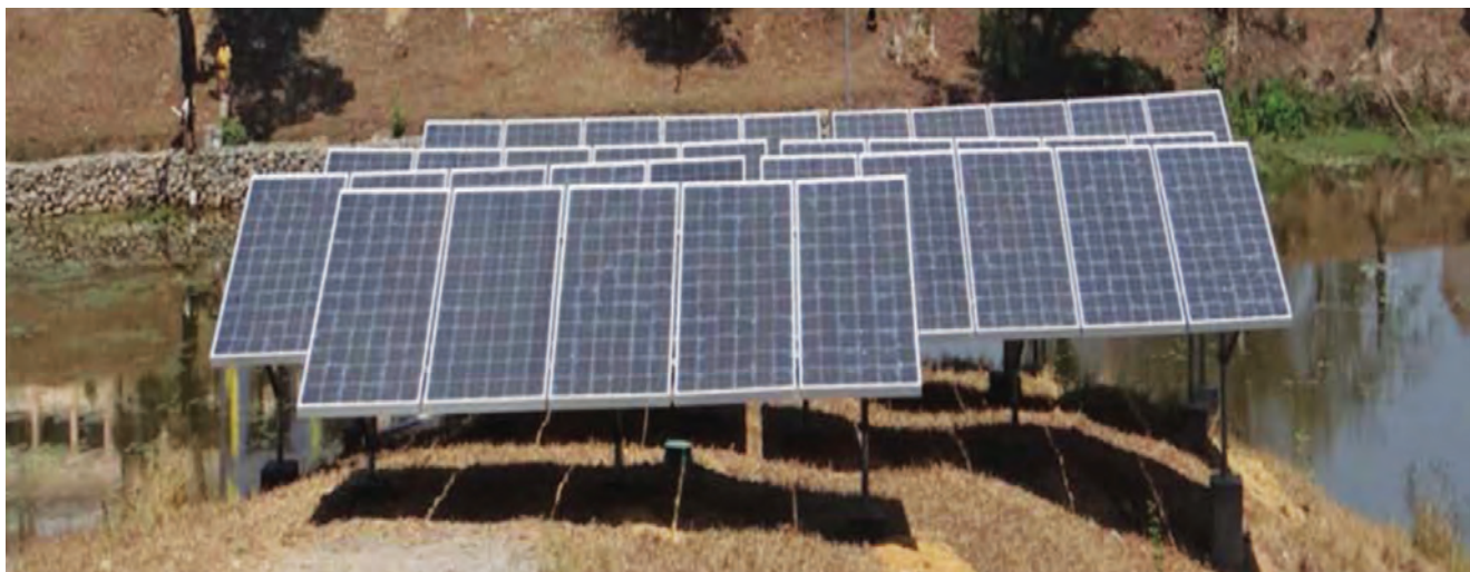
Solar panels inside campus
